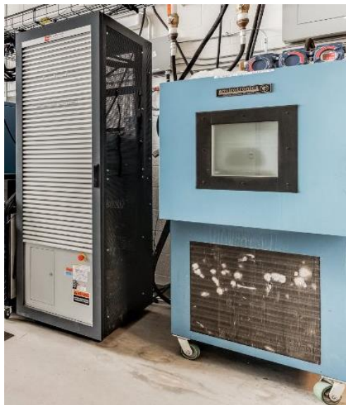
Figure 3.1: Digatron cycler (left) and Envirotronics thermal chamber (right)
