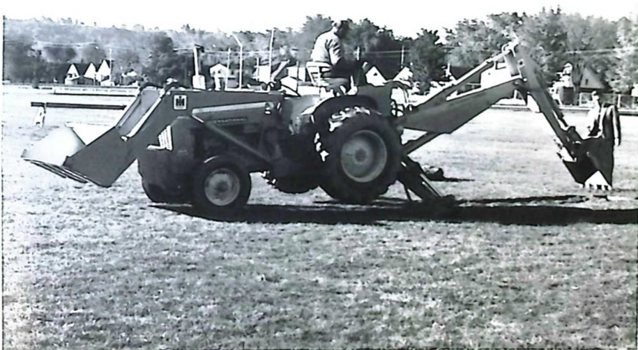
Plate 2. Mechanical shovel excavating pit. Note the flat, open aspect of the site.
