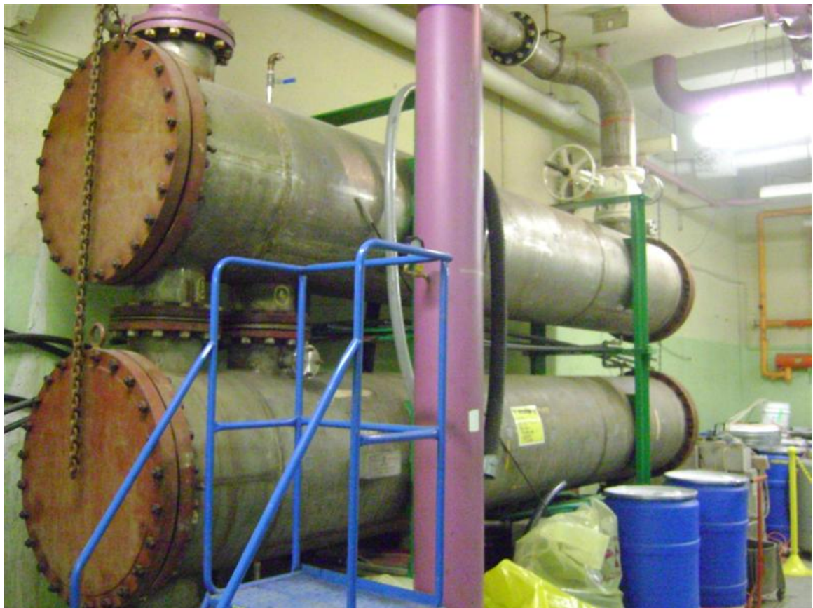
Figure 4.26: Picture of the two heat exchangers assembled in series.
