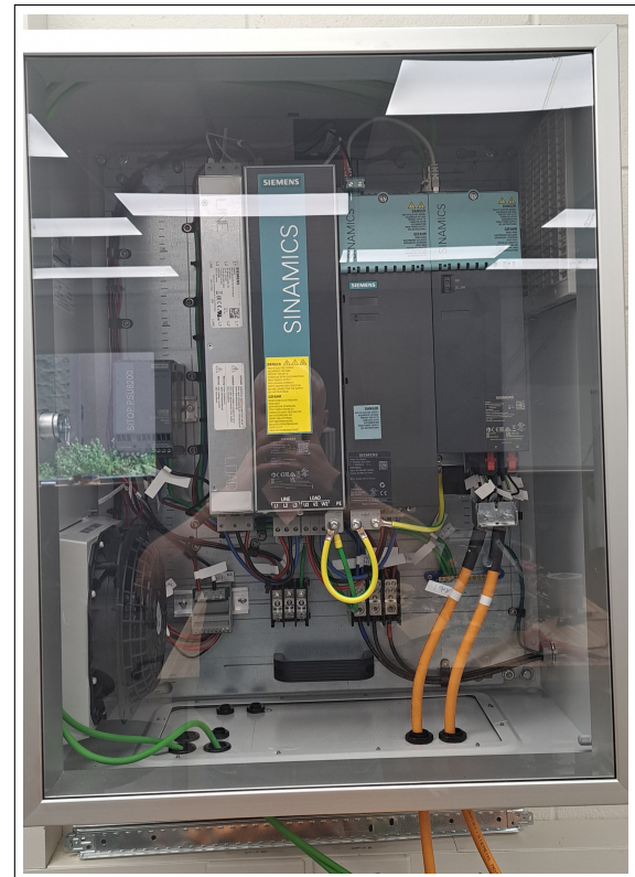
(b) High voltage motor drive cabinet
