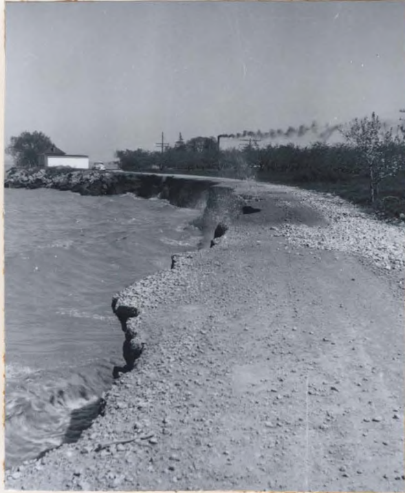
Fig. 31 A view of the road along the lake shore taken in May, 1951. It has been partly washed away but is still passable.
