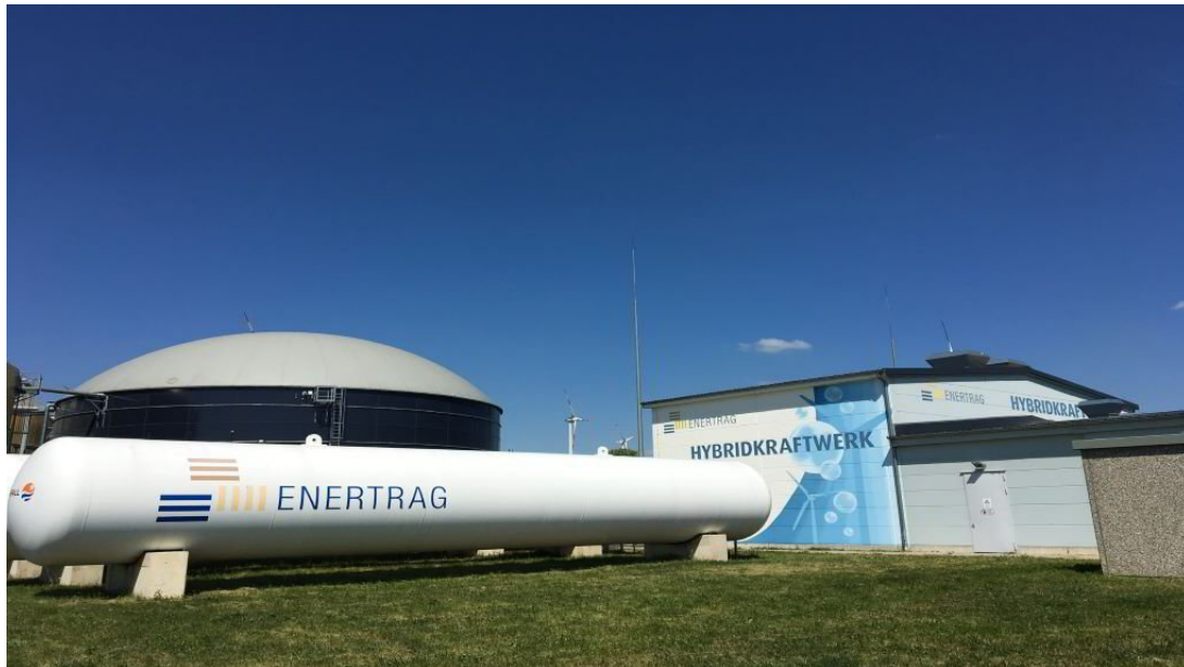
Figure 3.14. Hydrogen Tank at Prenzlau, Brandenburg in Germany [27]
