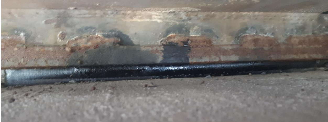
Figure 21: Bearing J2-W with unidentified liquid over the majority of bearing face
