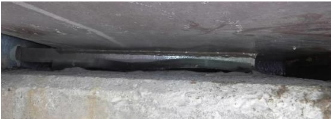
Figure 13: Unreinforced, failed Steeles Avenue bridge bearing
