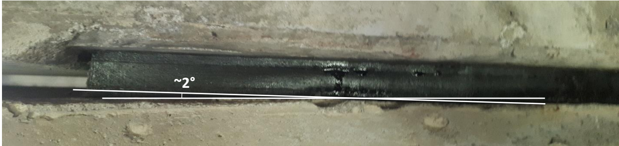
Figure 14: Damaged bearing at German Mills. Intersection point of white lines illustrates a change in inclination of the bearing of approximately two degrees, forming a 'bump' directly under the damaged region of the bearing.
