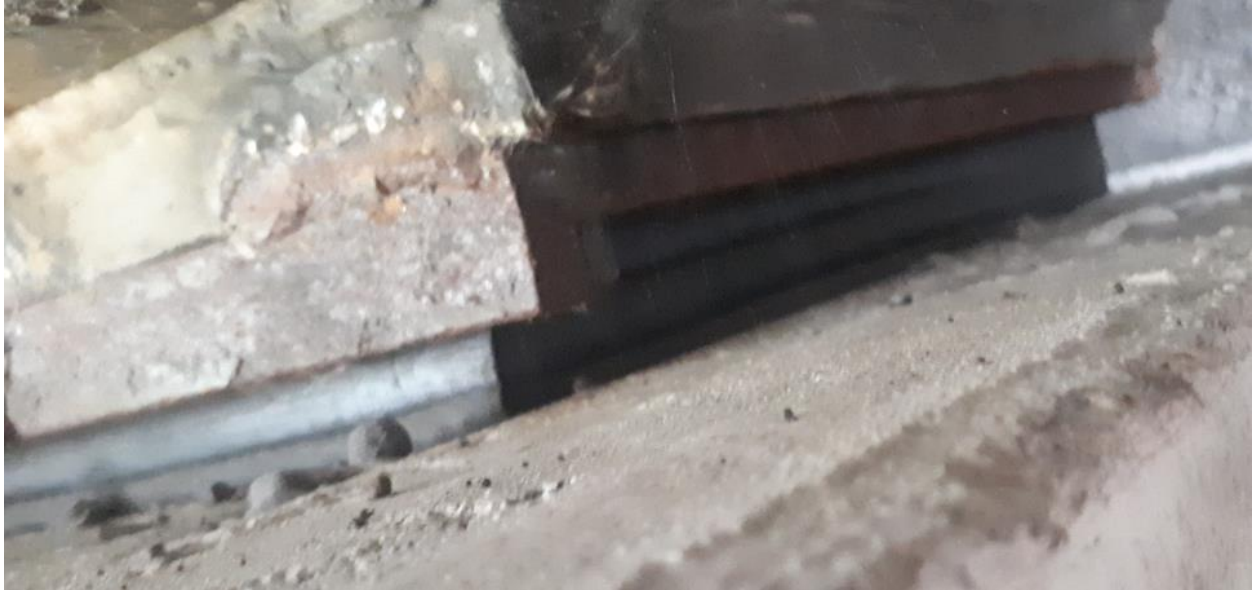
Figure 24: Bulging but undamaged bearing J3-E
