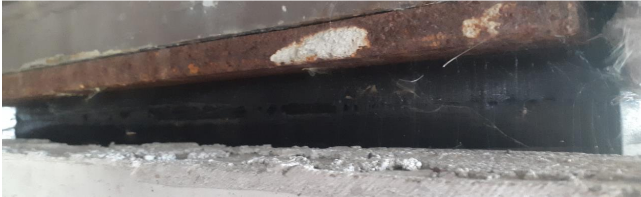
Figure 22: Bearing J3-W splitting behavior occurring along line of previous delamination
