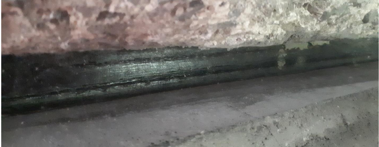
Figure 19: Undamaged bearing at German Mills Creek; slight bulging which is not indicative of damage
