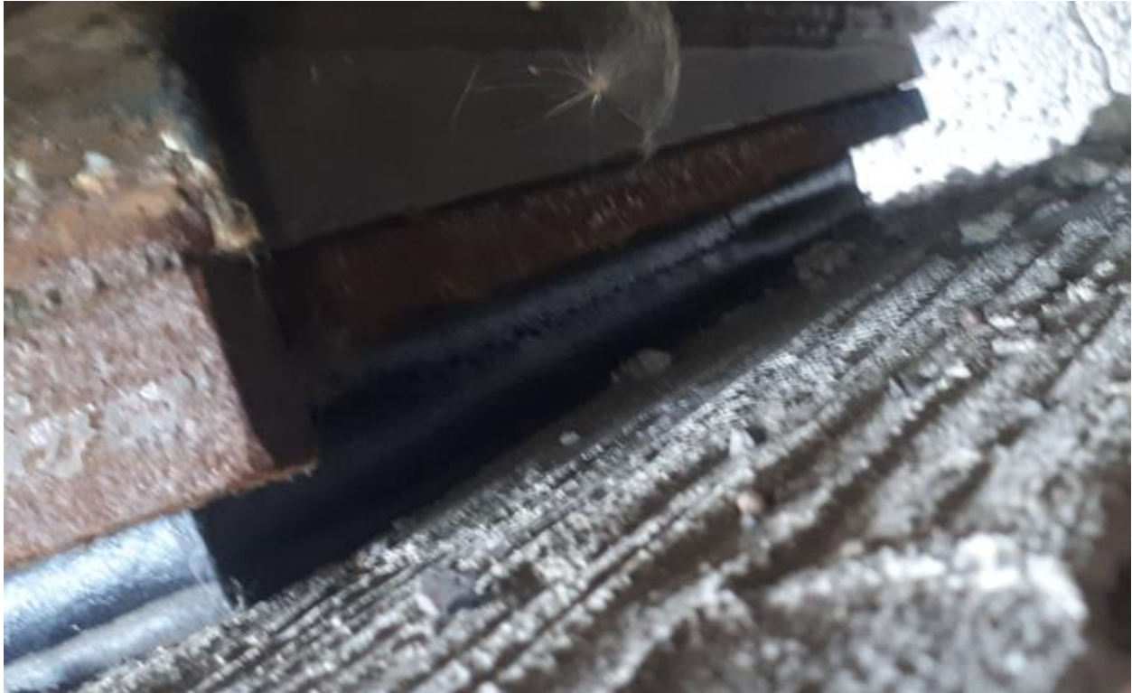
Figure 23: Limited delamination observed at bearing J1-W
