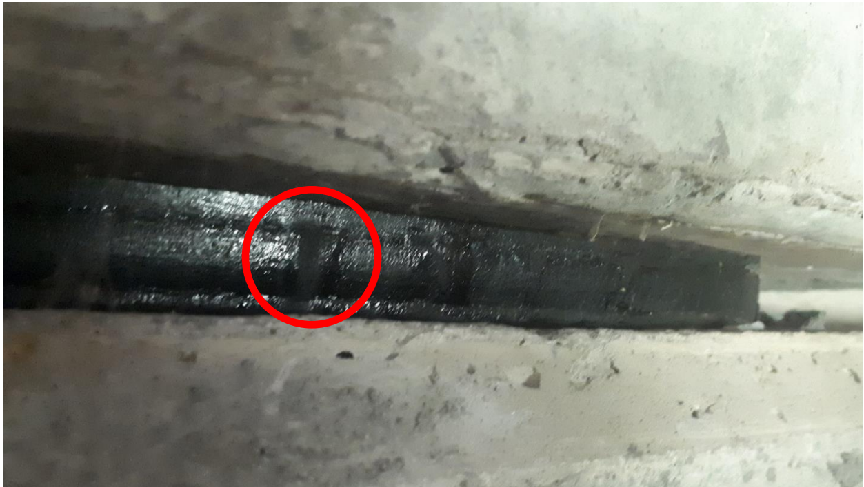
Figure 16: Bearing 1 at German Mills Creek site with location of liquid recovery marked
