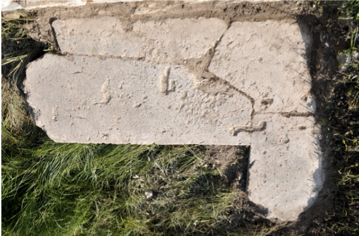
Figure 6b. Northeast corner of the Southeast Fountain House with Z-clamp cutting visible. Sourced from Paga, 2015: 359.
