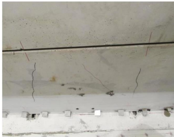
Figure 1.23. Specimen PFS2 cracks due to rebar discontinuity (Liu 2016).
