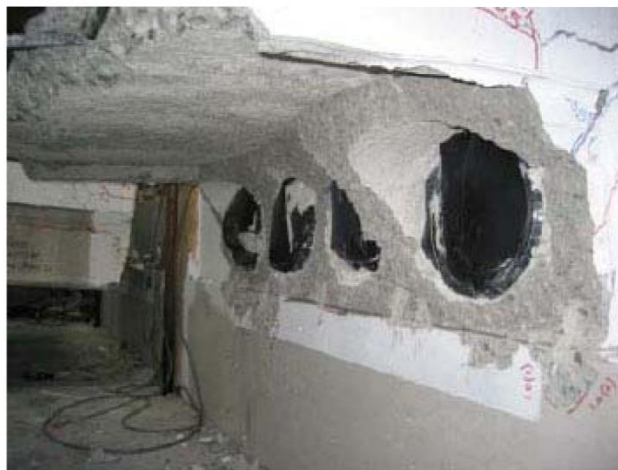
Figure 1.27. Flexure-Shear Failure (Bull and Matthew, 2003)
