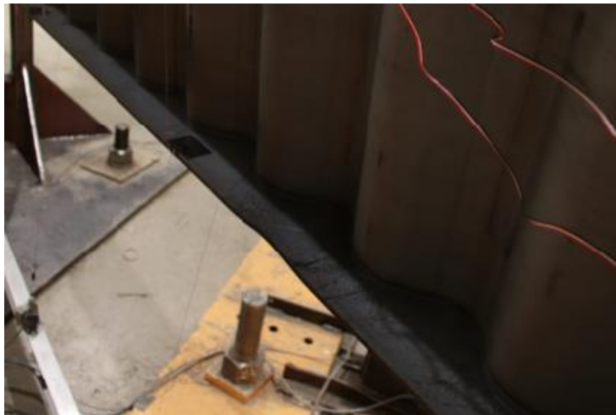
Figure A-13: Local Flange Buckling of the Deformed WTB333/127x6
