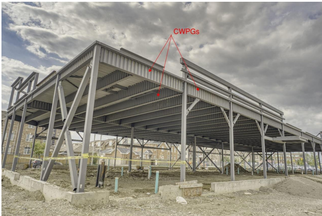
Figure 1-1: CWPGs in Commercial Building
