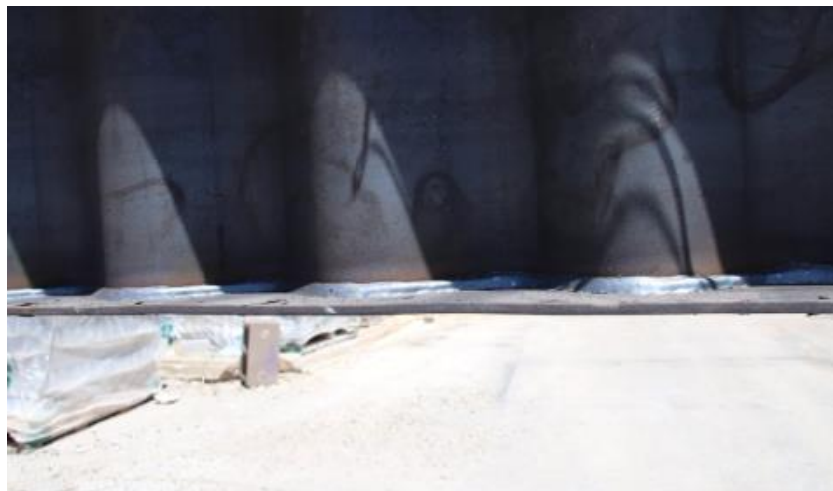
Figure A-17: Faint Local Flange Buckling of the Deformed WTF333/127x6
