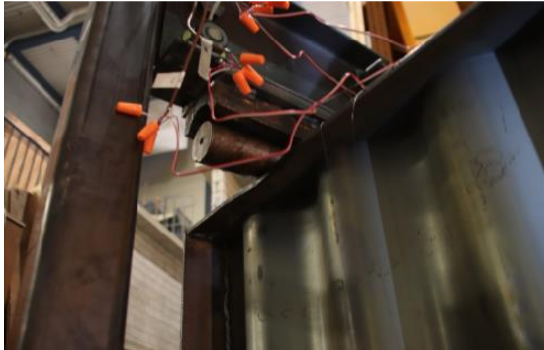
Figure A-7: Local Flange Buckling at Support of the WTA610/127x6
