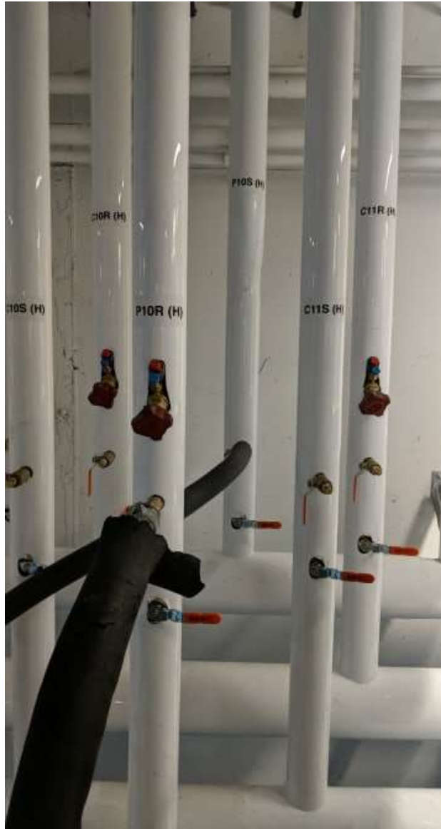
Figure 3.7 - Connection of the borehole string and GeoCube
