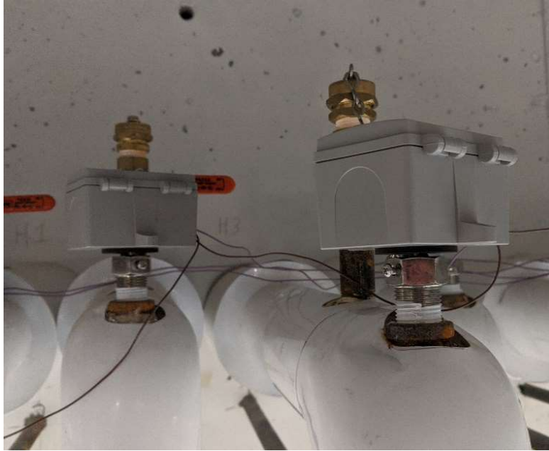
Figure 3.4 - Inlet and Outlet Thermistors
