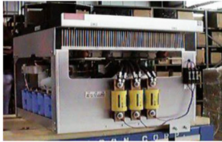
(a) Power Cell
