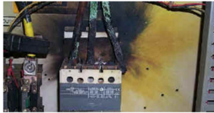
(c) Arcing Caused by Loose Contacts
