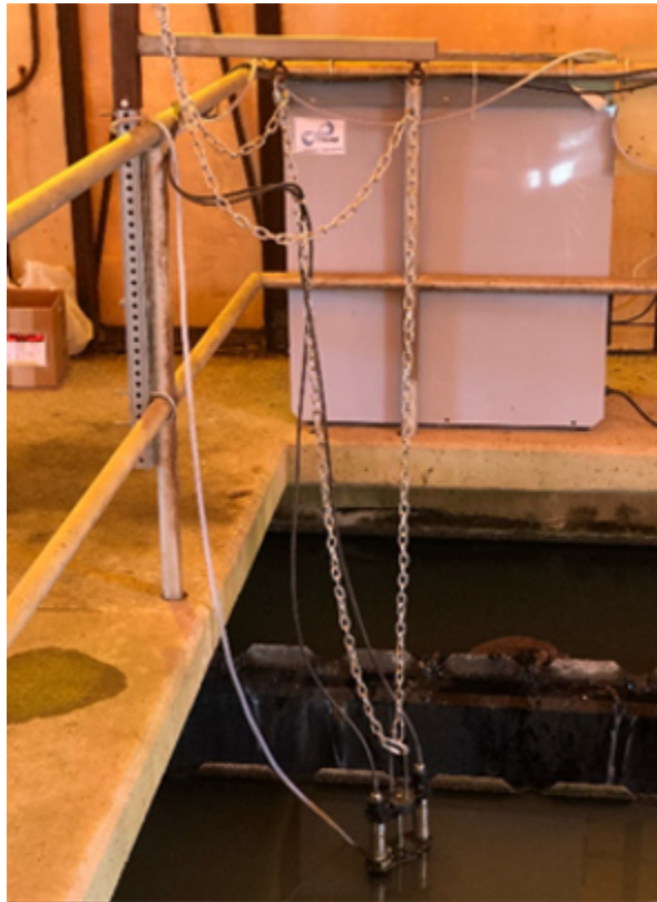
Figure 3.17: RSM30 Monitor Station at Dundas WWTP
