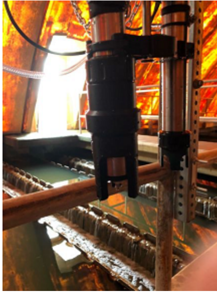
Figure 3.18: Sensors in the Dundas WWTP
