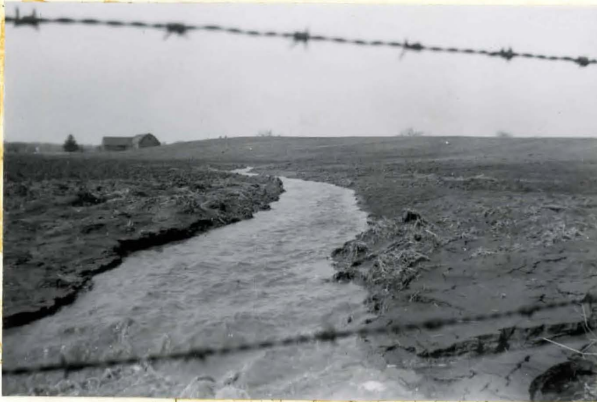
Photo 58. Swiftly flowing water in a drainage ditch. Erosion has started along the banks of the ditch. Grass lined ditches are recommended to cut down erosion.
