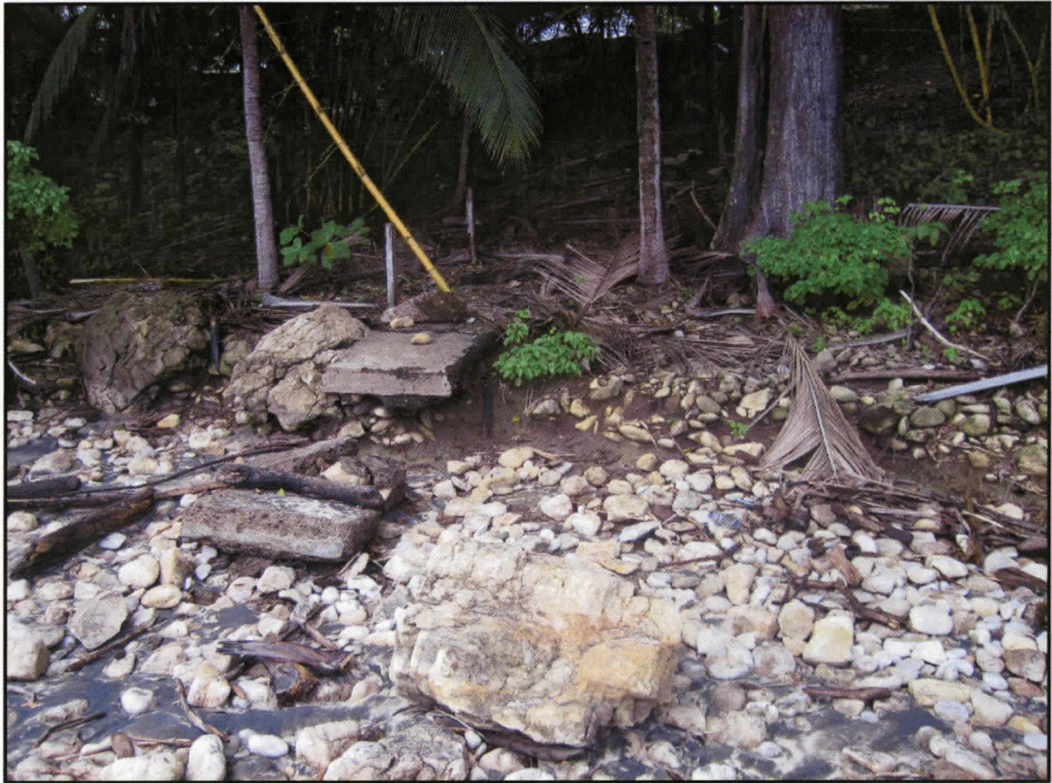
Figure 4.14: Evidence of relative sea level rise is evident by the erosion of this staircase found at Playa Pelada 150 m north of Playa Guiones.
