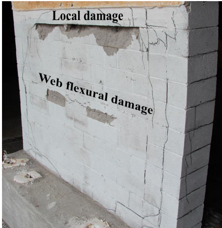
Fig 3.7. Local damage at web of Wall 7
