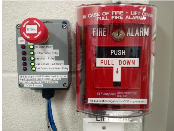
Figure 23: Energy storage lab emergency stop button and CO 2 fire suppression system pull station
