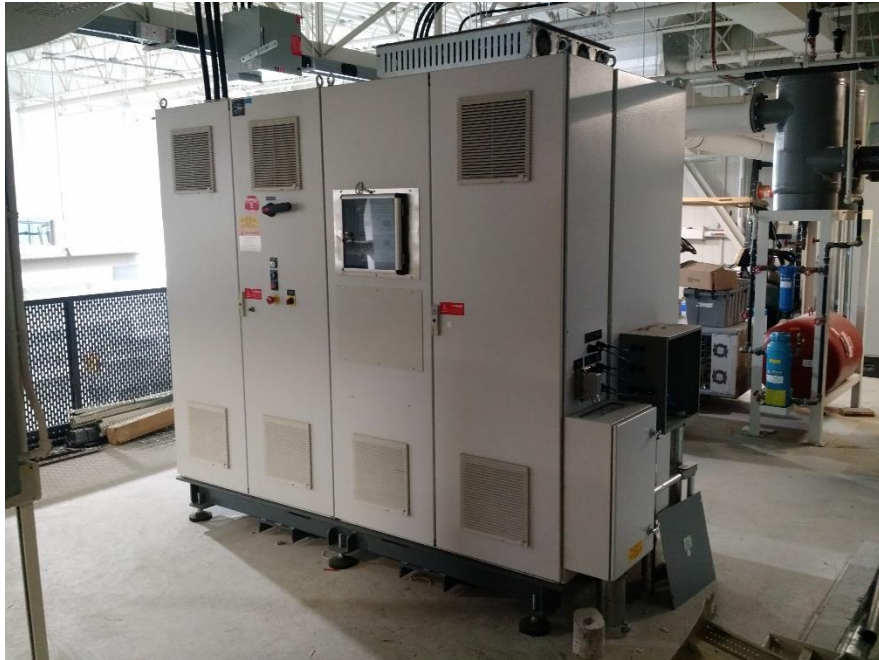
Figure 4: D&V Electronics BST240 battery pack testing equipment located in the mezzanine above the energy storage lab.
