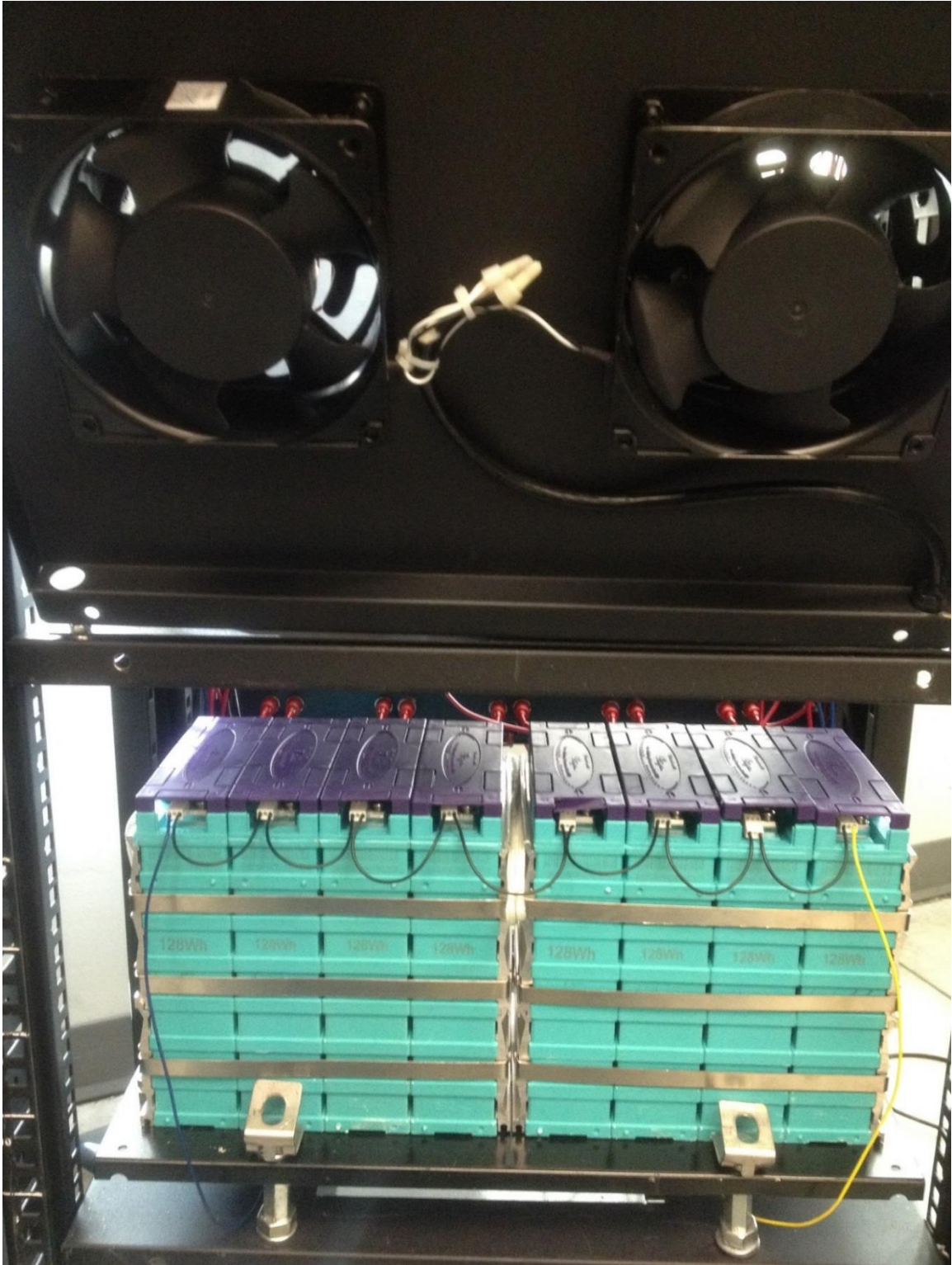
Fig. A. 2: HESS Battery banks and cooling fans
