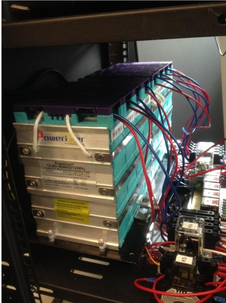
Fig. 5.10: Battery banks arrangement
