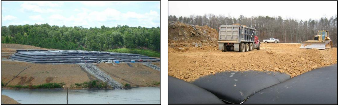
Figure 10. Images of geotextile dewatering bags filled with consolidated MFT. These tubes can be covered with aggregate material and vegetated as part of an oil sands reclamation program [34].
