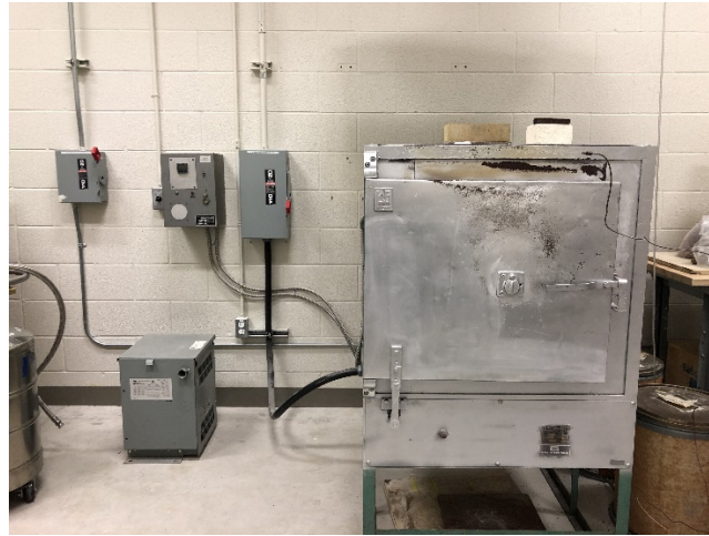
Figure 3.5. Furnace utilized O-temper specimens for heat treatments to attain.
