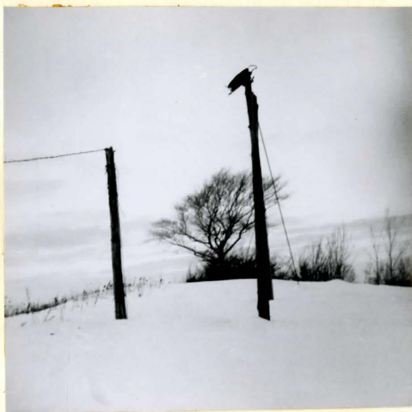
Photo 40. The broken ski tow gives evidence that the ski hills are no longer utilized..No tow rope is present and the pulley is twisted and broken.
