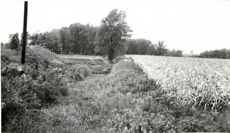
No. 27. Weed choked municipal drain needs cleaning. In the middle distance is a dugout pond used for irrigation. Ground water level is high on the sand plain. Con. V.
