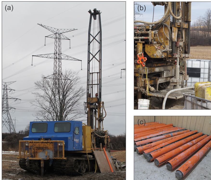
Figure 8: Field activities at the CTS: (a) a CME 75 track mounted drill rig used to core new boreholes at MW5-14; (b) extraction of the core from the subsurface via a wireline core retrieval system; and (c) 1.5 m long, PQ sized (85 mm) sediment cores placed in PVC core tubes awaiting sampling.
