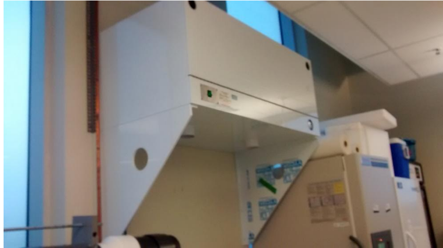
Figure B-12: HEPA Filtration System
