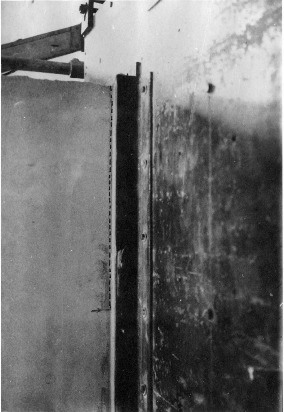
PLATE 7 CRACKING PATTERN ALONG THE BACK WALL OF BUILDING 1
