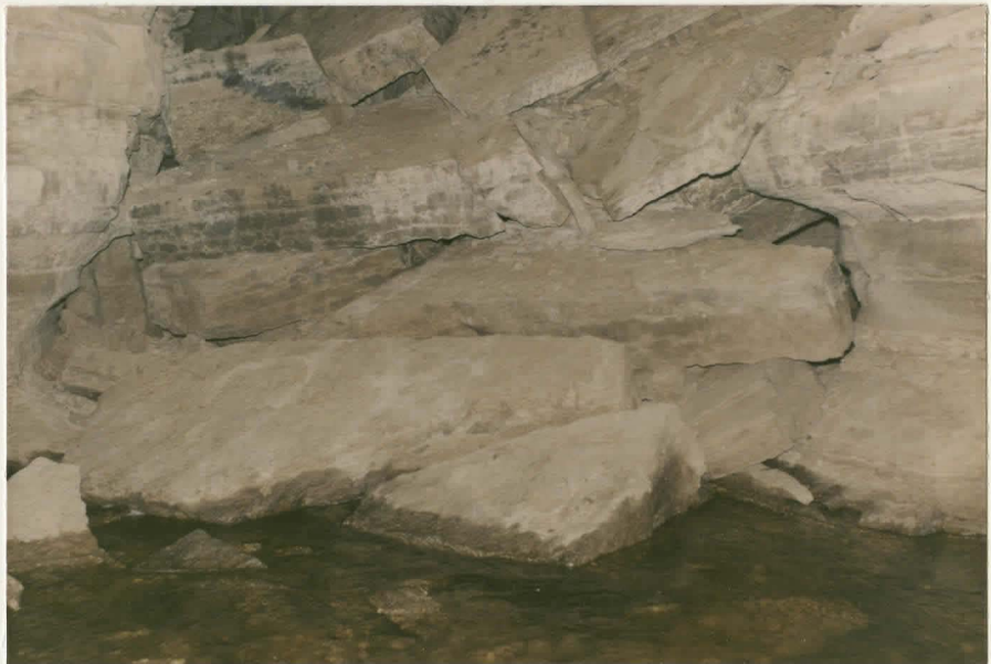
PLATE XI: Collapse at Karst Window No. 2, from inside the caves
