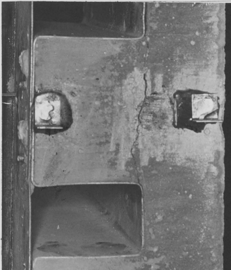
(a) Cracking of Concrete Rib
