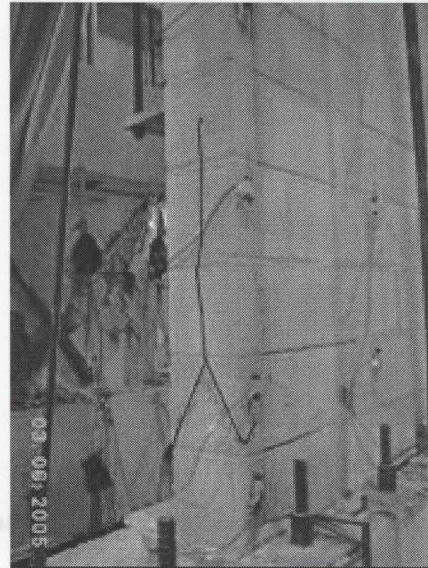
(b) East toe cracking
