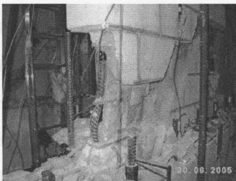
(a) Bar buckling (East)
