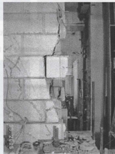
(b) Spalling of end blocks
