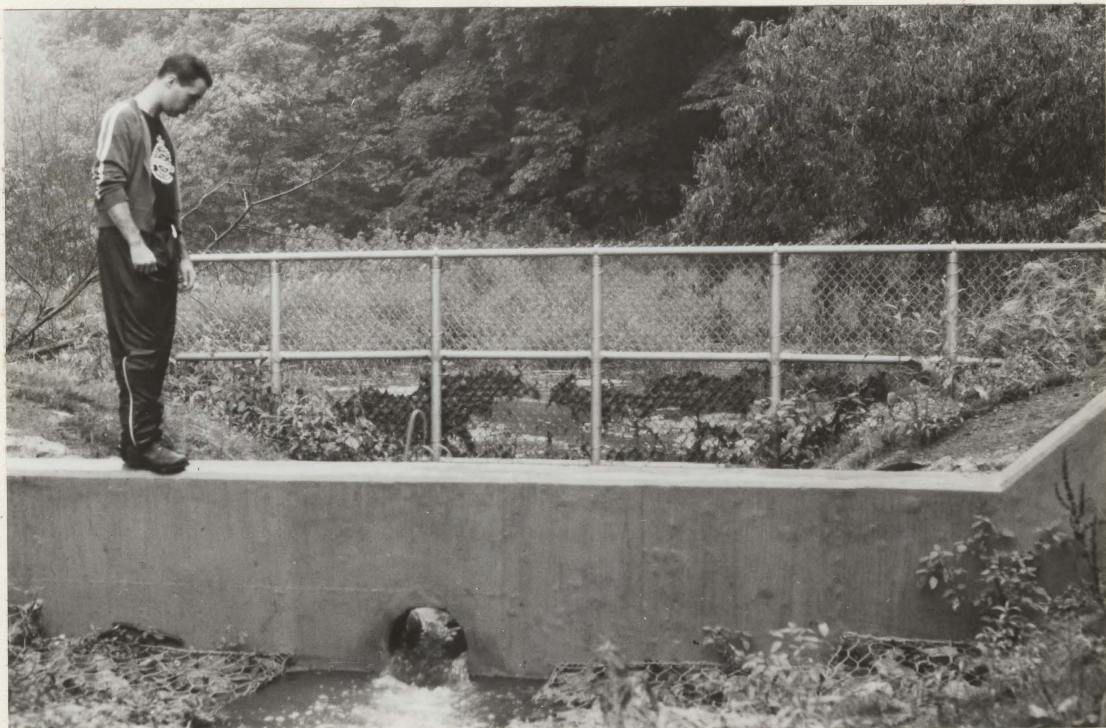
Figure A1.2 The stormwater detention pond's dam early in August 7/86 storm event.
