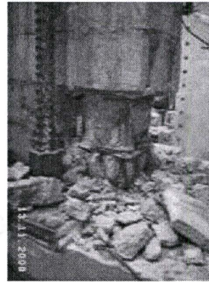
b) Spalling at the left toe
