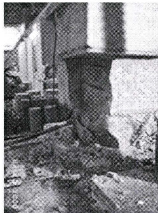
b) Spalling at left toe
