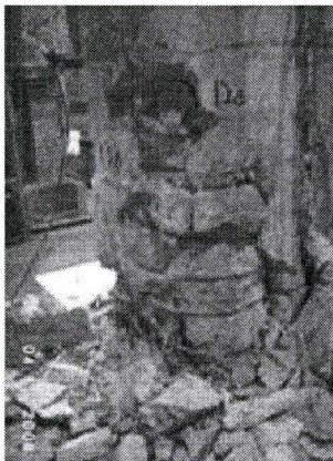
a) Broken spiral at right toe
