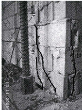
b) Inclined cracks (right)
