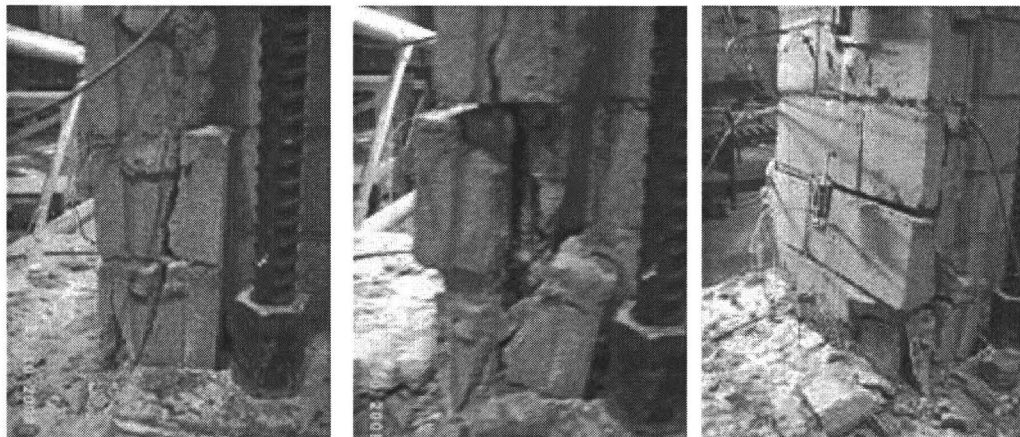
a) Widening of cracks b) Grout column splitting c) Spalling of face shells
