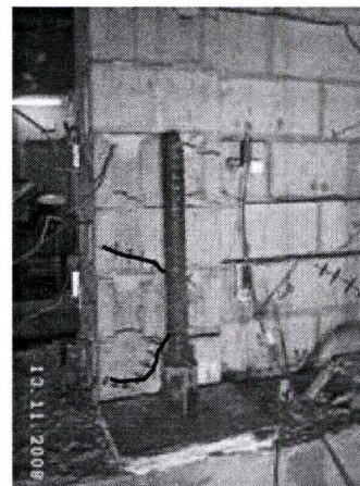
c) Inclined cracks (left)
