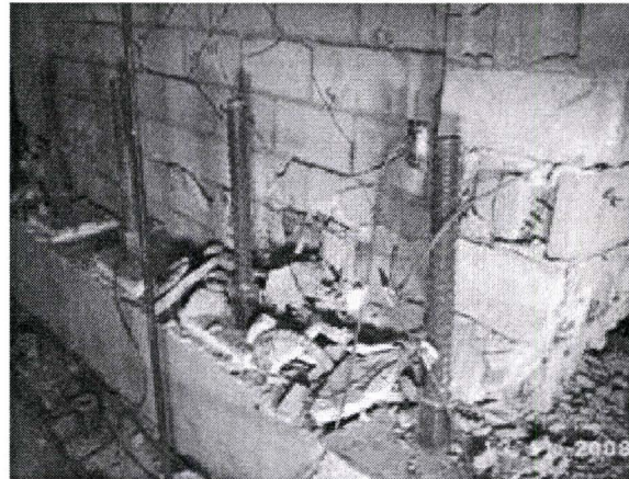
d) Deterioration of the second course
