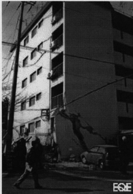
Figure 2. 1 Premature shear failure of Structural wall, during 1995 Kope, earthquake. ( http://www.hewett.norfolk.sch.uk/curric/NEWGEOG/Tectonic/Earth/Building.htm (accessed March 2006))
