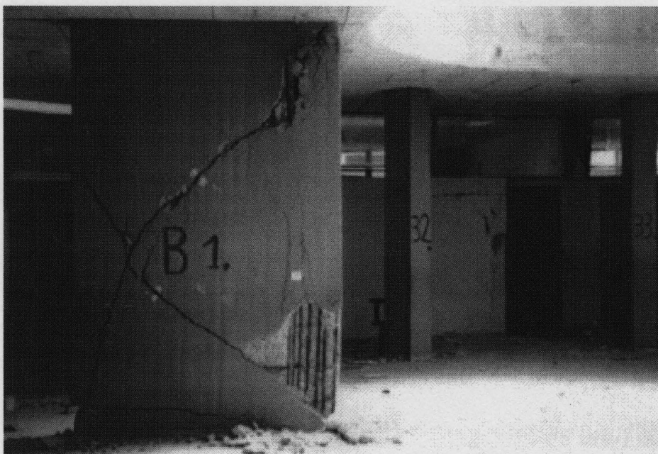
Figure 2. 2 Failure of a structural wall during the 1986 Kalamata earthquake (Lopes 2001).
