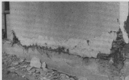
Figure 2. 4 Failure of shear wall observed after the 1985 Chile EQ. (Wyllie et al. 1986).
