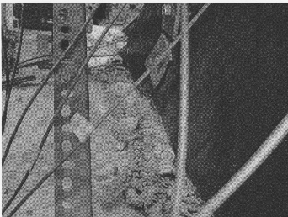
Figure 4- 57 Concrete crushing at the bottom of wall RW7.
