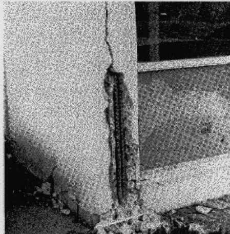
Figure 2. 3 Failure of a structural wall construction joint during the 1971 San Fernando EQ. (Jennings 1971).
