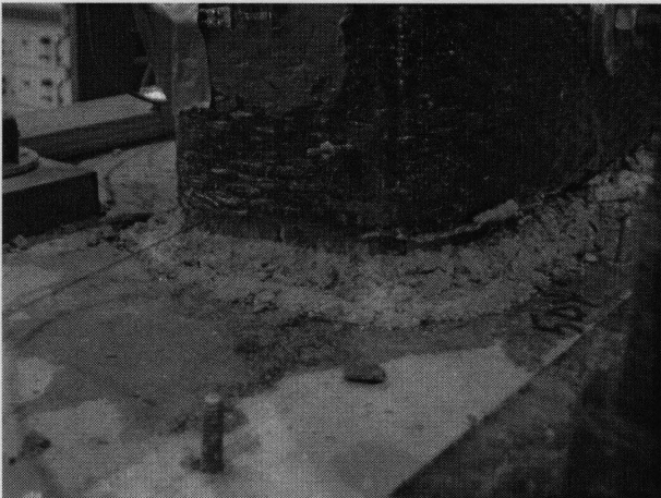
Figure 4- 16 RW3 at failure.
