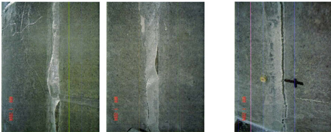
(a) Concave Bed Joints Not Completely Filled with Epoxy (b) Concave Bed Joints Filled with Epoxy
