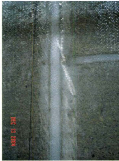
Figure 3.22 – Minor Damage to GFRP Along Bed Joint (Prior to Full Fabric Tearing)
