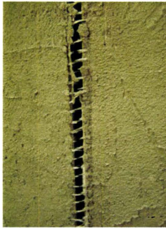
Figure 4.3 – Typical Fibre Damage (Tearing) of Bed Joints Reinforced with 4.5 oz. Mesh at 0^{\circ}/90^{\circ}
