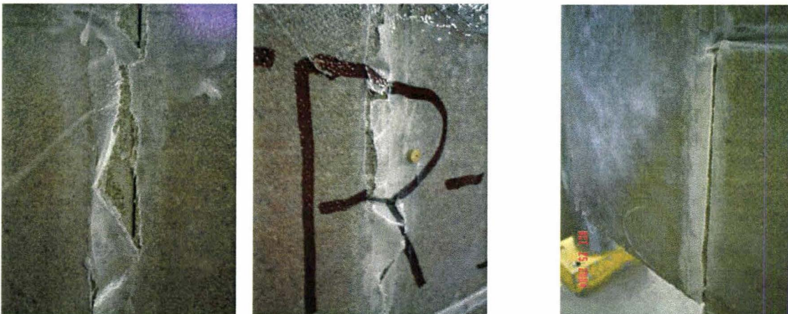
(a) Concave Bed Joints Not Completely Filled with Epoxy
