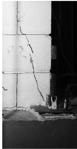
a) Vertical Toe Crack at 34.5 mm Cycle
