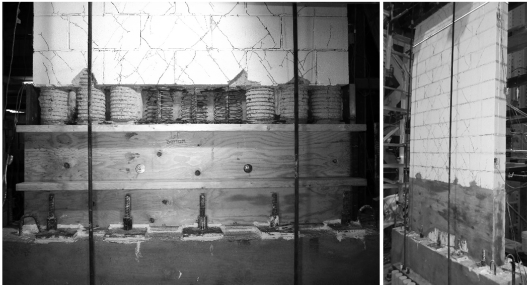
a) Formwork for Repair Grout Pour, Showing Open Fourth Course for Initial Pouring b) Repair Grout Following Removal of Formwork
