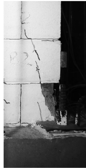
b) First Spalling to Reveal Confining Device at 46 mm Cycle
