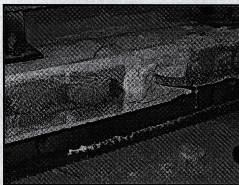
Figure 3.16 – Effectiveness of the plastic mesh in preventing grout flow to the lower courses (picture taken after demolishing the tested shear wall specimen)
