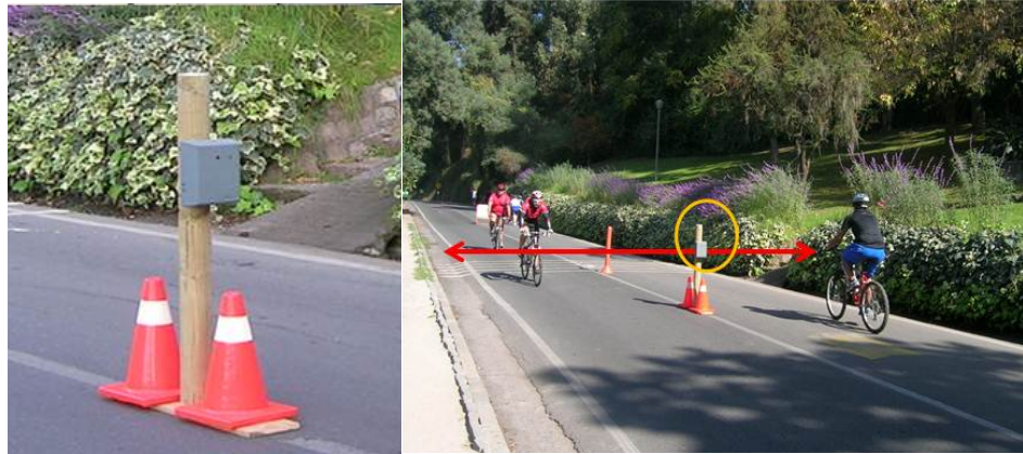
Figure 32. Pyro Box Compact Device Installed in measuring point P1
