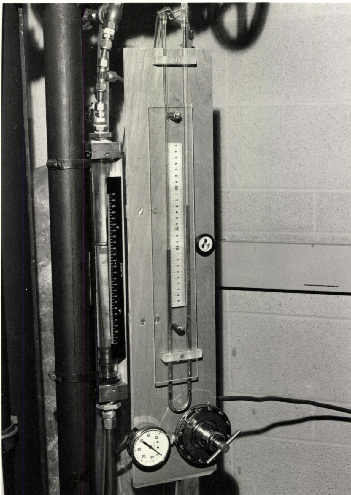
Plate #3 Polymer injector controls and flowmeter
