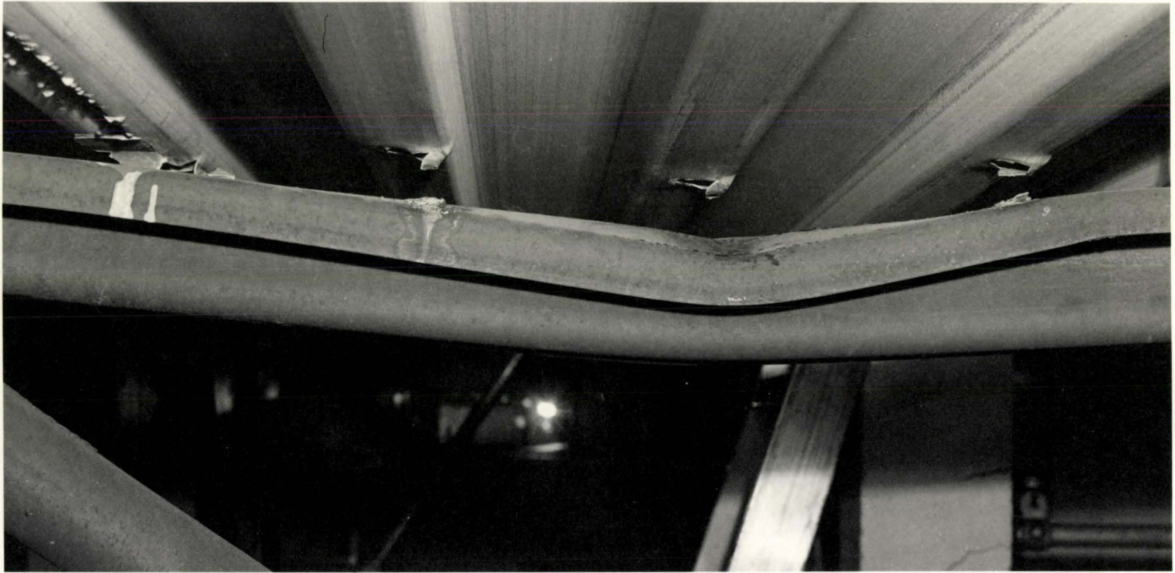
FIG. 3.6 FAILURE OF BEAM III
