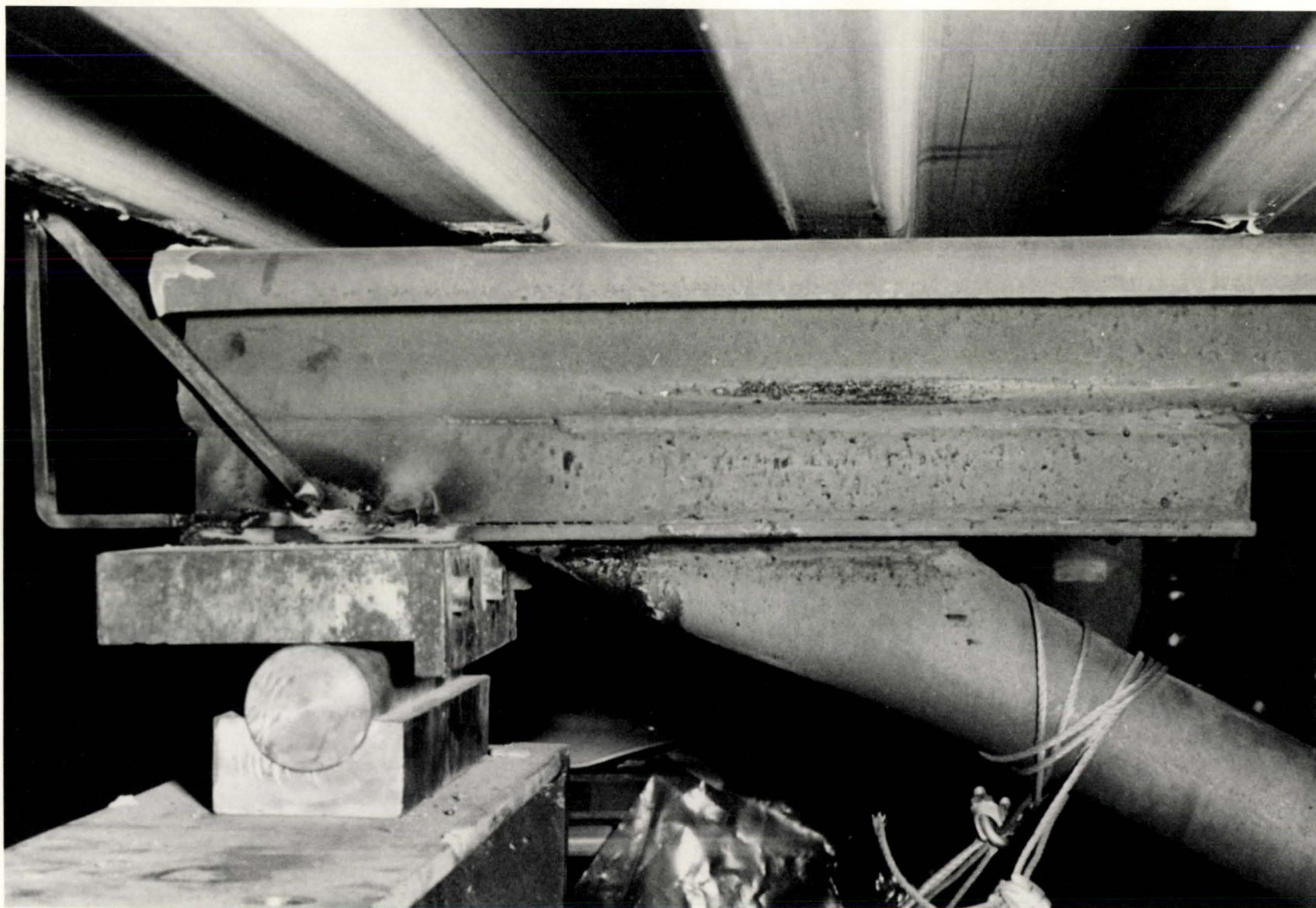
FIG. 3.5 FAILURE OF PUDDLE WELDS AT SUPPORT
