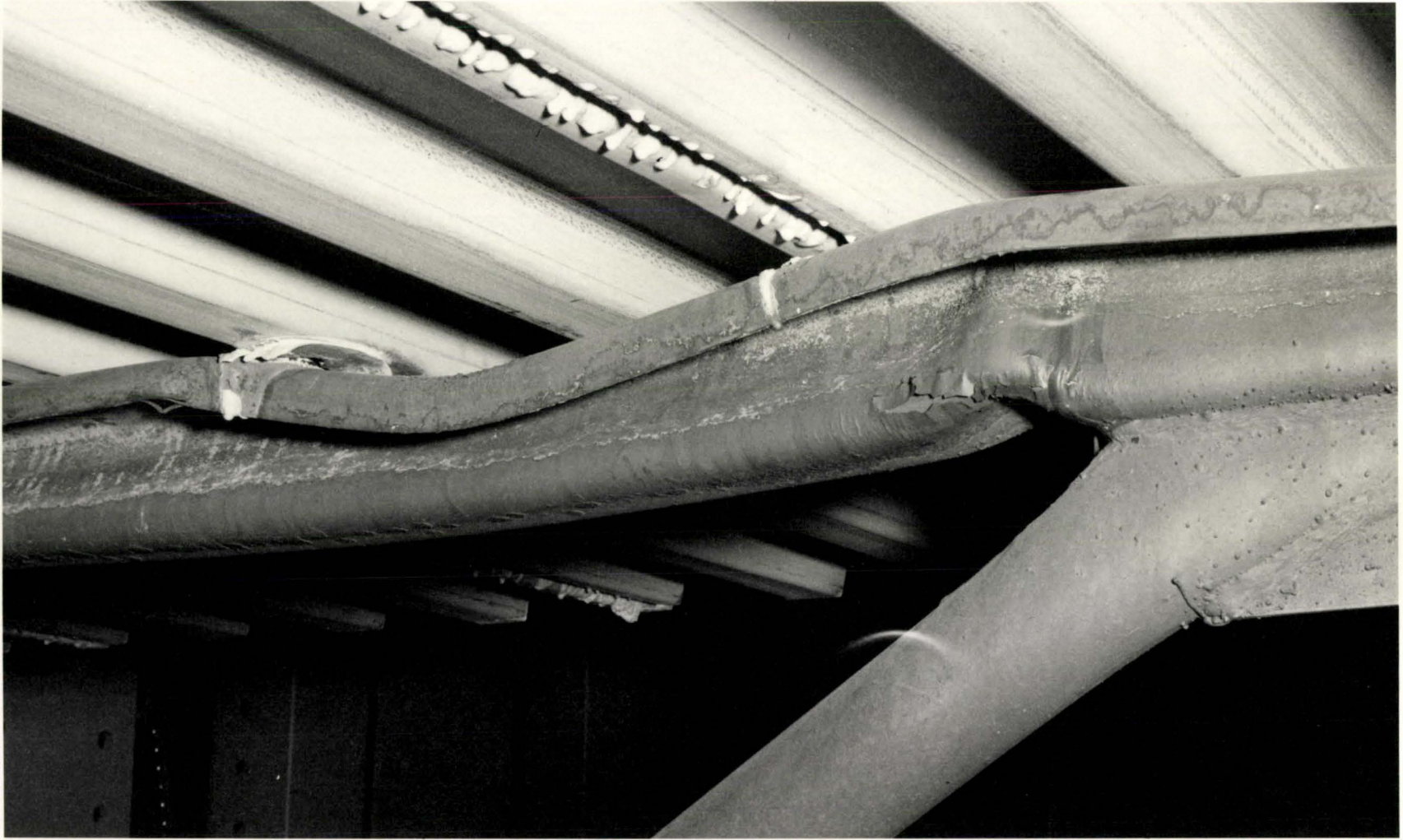
FIG. 3.4 FAILURE OF BEAM II
