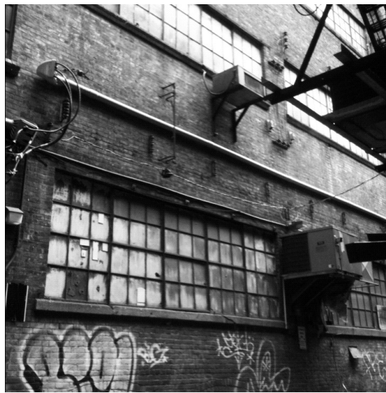
Figure 5.9 Graffiti, broken windows, and electrical work in “Crack Alley” (Author, 2012)
