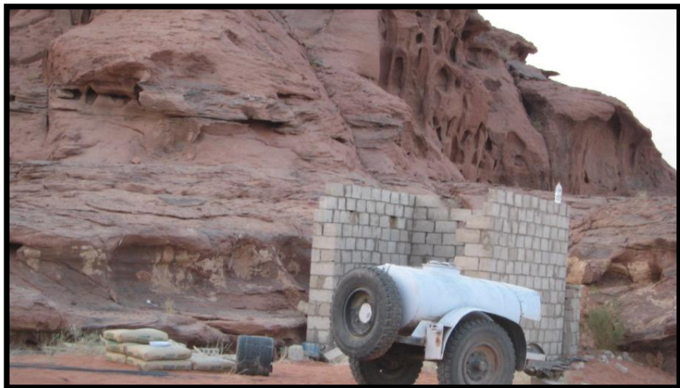
Photograph 6 The beginnings of a new USAID toilet for Lawrence Camp in the WRPA.
