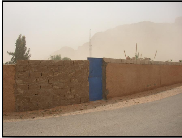
Photograph 9 Bedouin modifications to one of the village walls. The owner took it upon himself to fill in a large opening to the left of the door. Additionally, the wall to the right of the door has had a row of cinder blocks added to give the wall height so that no one passing by can look over the structure.
