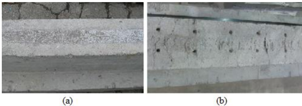
Figure 4.34: EBA2 (a) After the chiseling away of excess epoxy and (b) With significant cracks from previous testing
