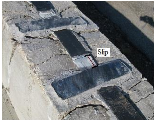
Figure 4.36: Slip in debonded FRP in EBA2
