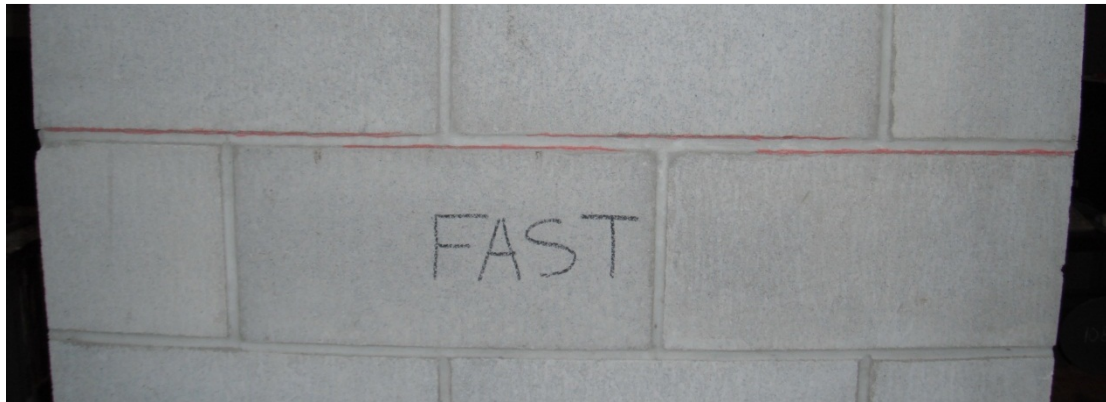
Figure B-0-3: Close-up of Initial Crack Pattern at a Deflection of 2.5mm of B-1 2.2m Wall
