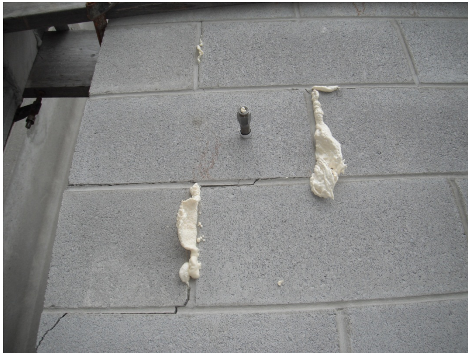
Figure B-0-28: Pre-mature Failure of B-2 Wall With Three Roped Cells Due to Expansive Force of the Foam
