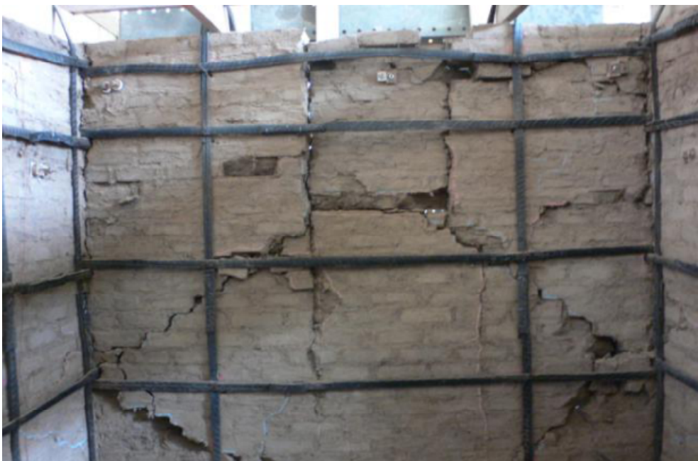
Figure 2-13: Damage to Rear Wall of Structure After Severe Shaking (Charleson, 2009)
