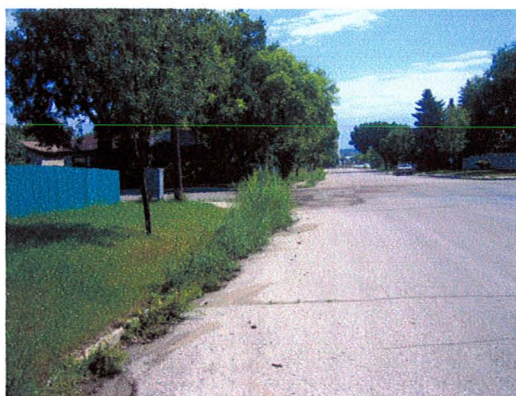
Image 35: View of Overgrown Curbs
